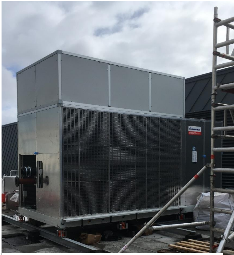
Figure 2 HRI ED Air Source Heat Pump prior to install and commissioning
